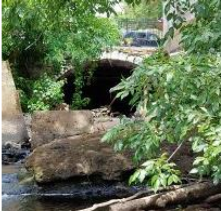
Along side of Mill #3 looking west at east end of the east bridge section
