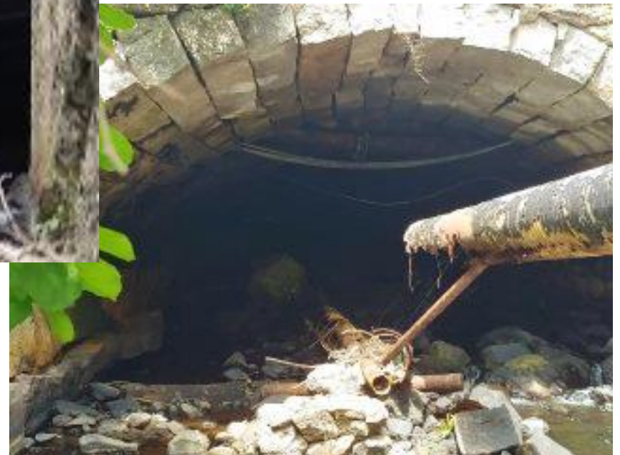
At entry to east bridge the pipe is completely broken off. Electric cables can be seen hanging down inside
