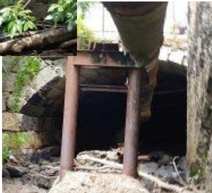
Along side of Mill #3, with steam pipe support, looking at left arch foundation.
