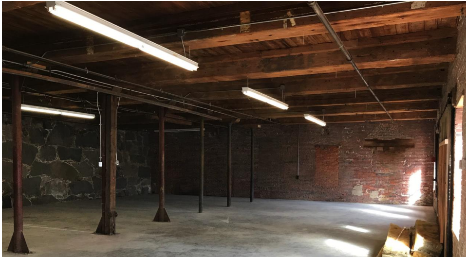
The lower level of Mill 2 – brick, stone, iron and wood are prominent materials. The beams are single pieces of wood – each over 50 feet long. (photo by John Mayer)
